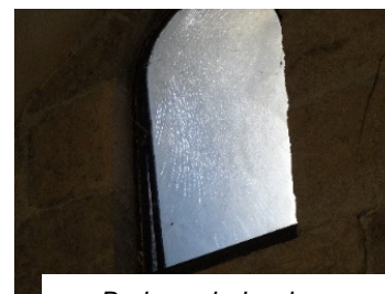
Broken window in Damascus Citadel
