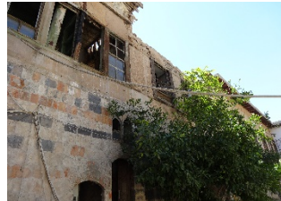
Damaged wing of a building
