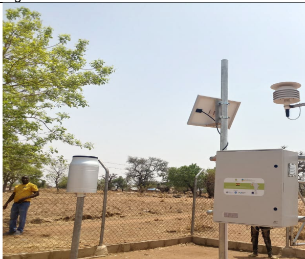
Figure 4: Installed meteorological station
