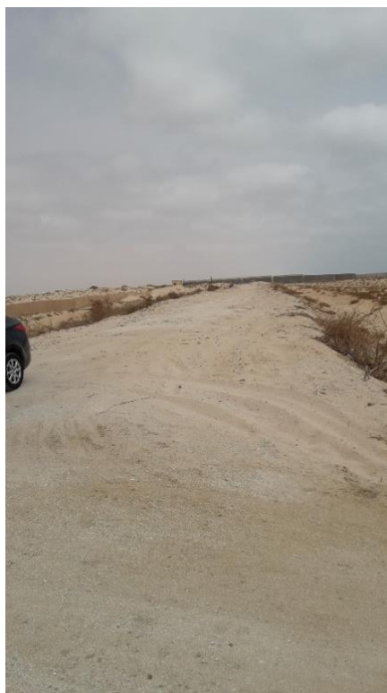
Figure 15: Vegetation on protected coastal dune bulldozed as access road to building site, July 2019
