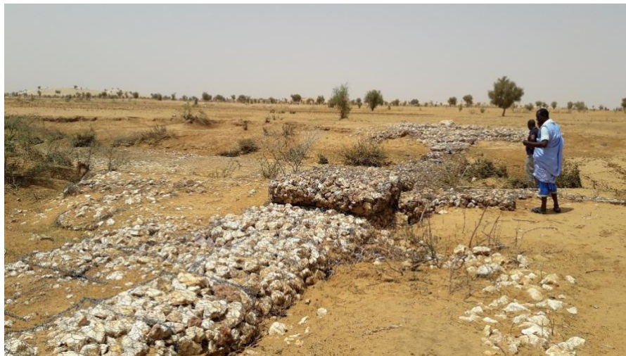
Figure 7: Beilougue Litama Block dam, installed 2014, still functioning, cropping area with shrubs in background (time 11.38.05)
